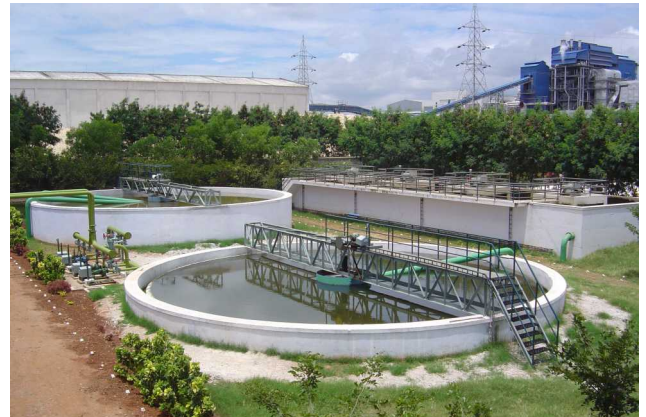
Sugar Plant ETP at Nanjangud – Karnataka
