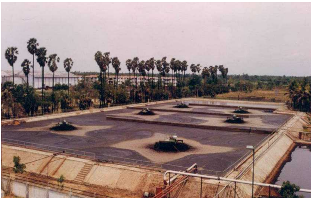
Distillery ETP at Thiru Arooran Sugars, Tamilnadu
