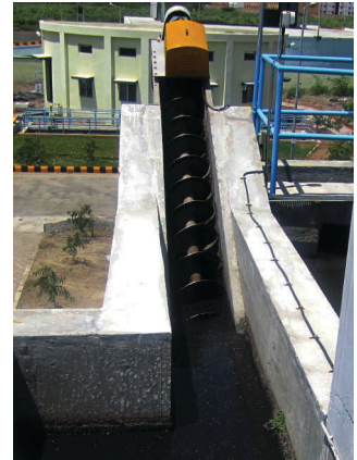
Screw Classifier Assembly Nagole STP, Andhra Pradesh
