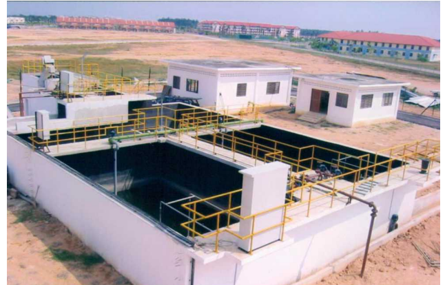
STP at Parit Bunter – West Malaysia
