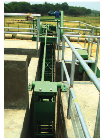
Rake type Classifier Assembly 50MLD STP, Chandigarh
