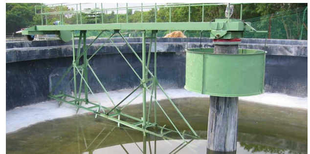
Type SPC-B 21m dia Peripheral driven Traction Clarifier at Crimson STP, Malaysia.
