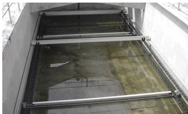
Type SP-STD: Rectangular Clarifier, Kuantan STP, Malaysia
