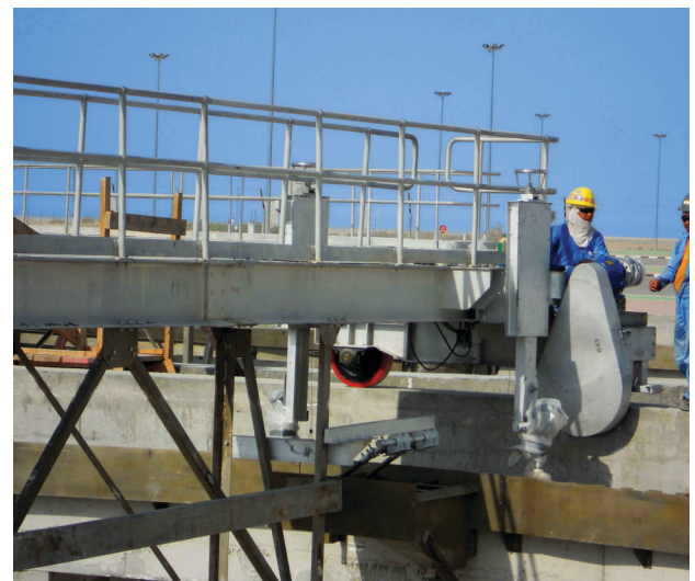
Type SPC-B Peripheral driven Traction Clarifier drive assembly, Skimmer Assembly and Weir cleaning device – Doha STP , Qatar
