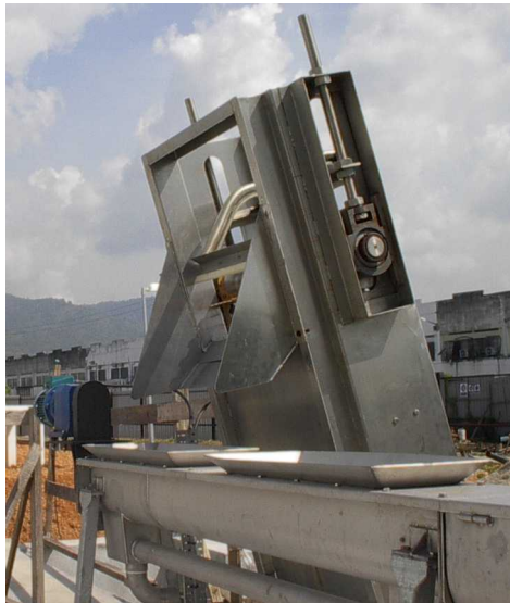
Type SP-M2-C Mechanical Fine Screen Biotropic Engineering STP, Malaysia
